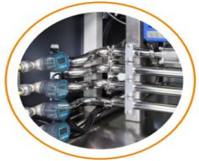
Cooling pipes and vacuum system pipes
