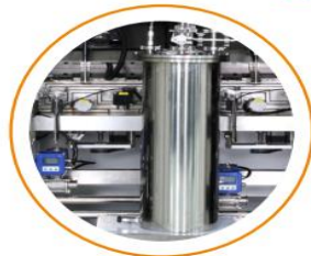
Formic acid control and protection system
